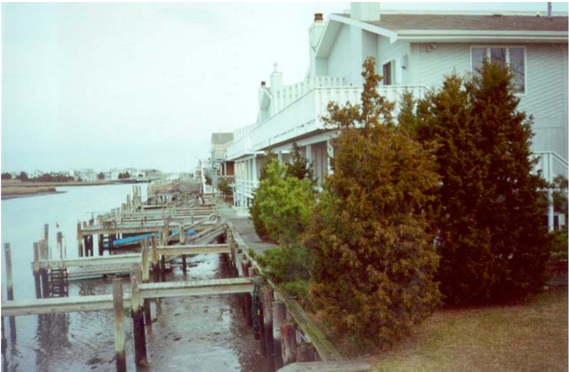
View north from the 30 th Street Bridge showing rear decks approximately five (5) feet from the bulkhead. Note the background where a deck is directly atop the bulkhead.
